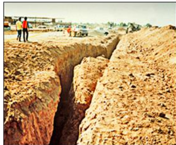
Figure 1 Excavation Cave In
